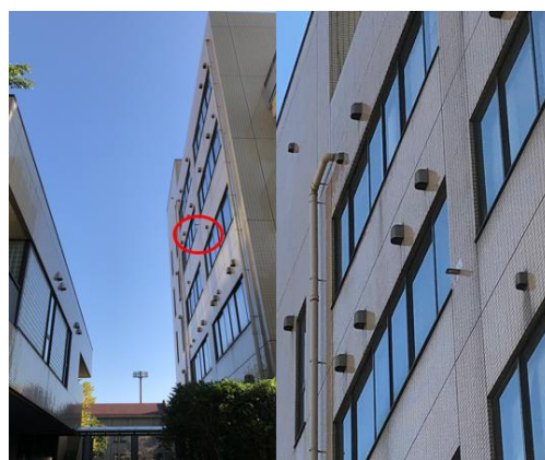
Fig. 13. Installation Status (northeast)
