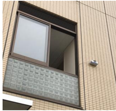
Fig. 8. Installation status (SE)
